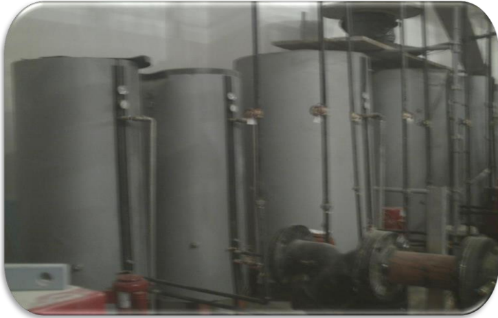
Hot water storage tanks
