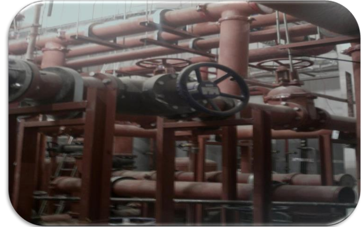
Chilled Water Piping in Pump Room
