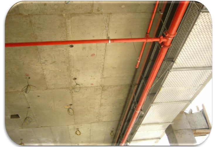
Fire Fighting Pipes and Cable Tray
