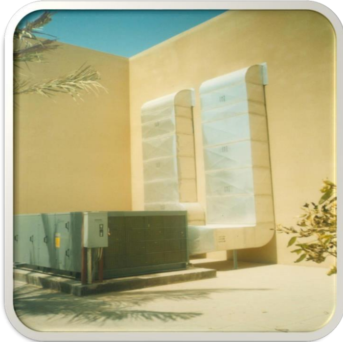
Out Door Ducts & Package AC Units
